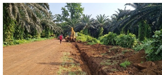
Figure 22: Rehabilitation route of the community of Ribeira Peixe
